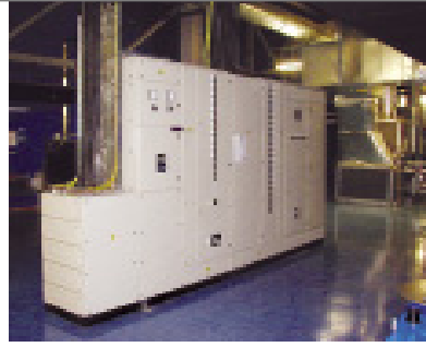
Electrical intake equipment. Ster Century, Romford.
