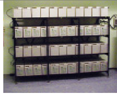
Emergency battery room. Warner, Islington
